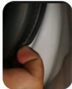
Left rear door frame edge sealing
